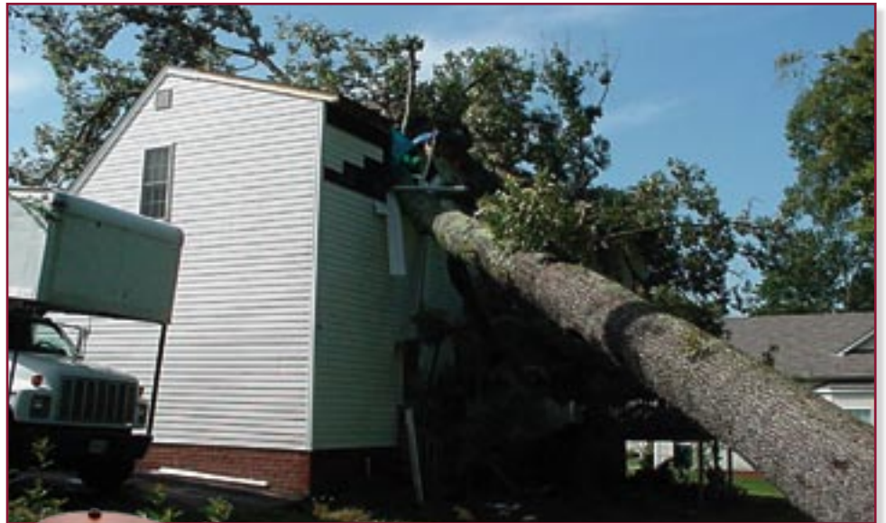
One of a number of homes damaged during Hurricane Isabel
